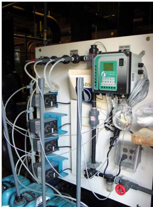
By helping design and specify water treatment systems such as this state-of-the-art cooling water treatment system, IWTP staff help participating state facilities.
