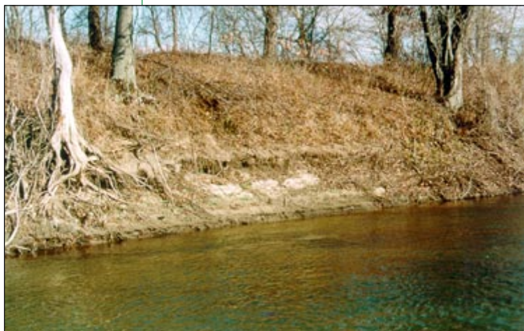
Erosion occurs along a bank of the Kankakee River.
