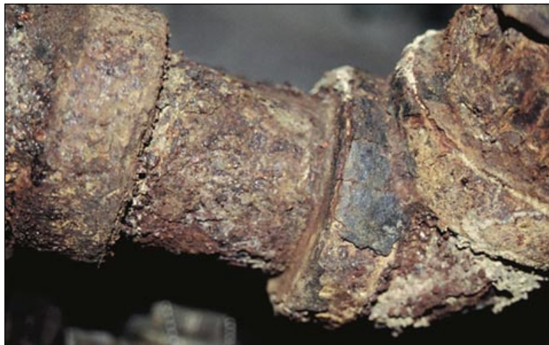
Here's an example of corrosion found under the insulation in the cooling system at a state facility.
