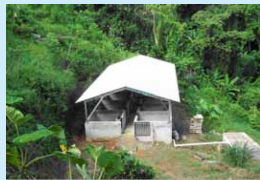
Demonstration animal waste management facility at a small swine operation in Rio Piedras, Puerto Rico
