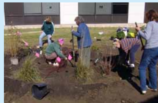
Master Gardeners construct a demonstration rain garden in Gloucester County, New Jersey
