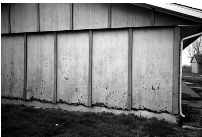
Decaying siding is representative of conditions found in apartment complexes managed by the realty company. OIG photo.
