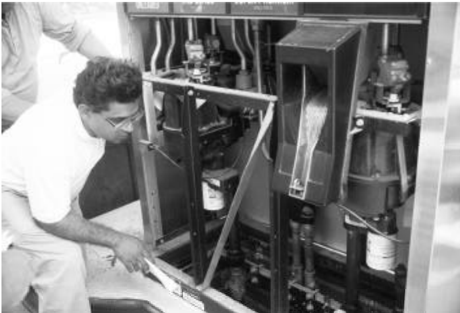
Inside the Pumps
