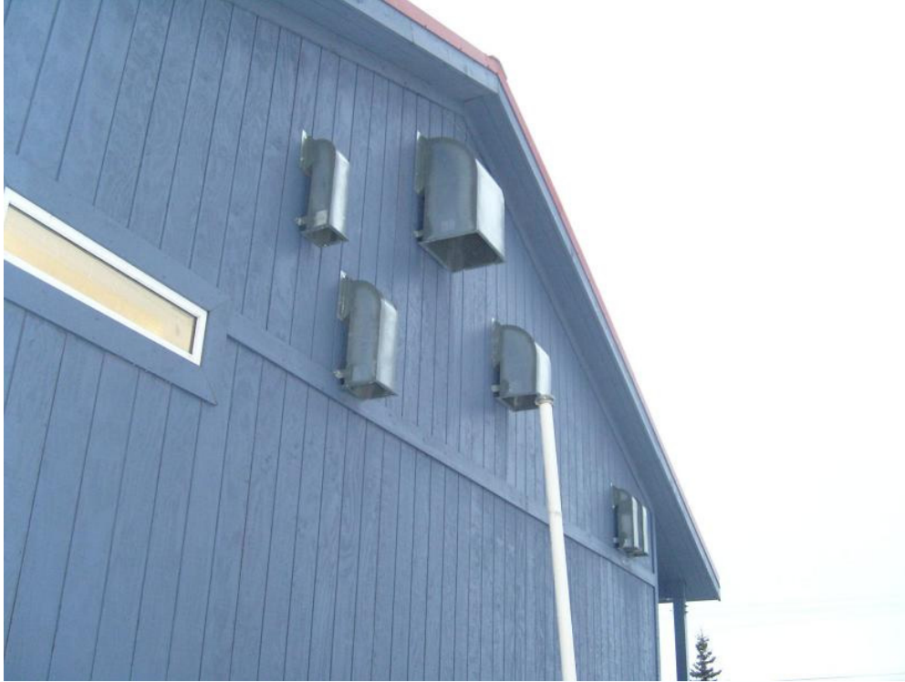
Exterior ventilation ducts on the north side of the Tuluksak Youth and Multi-Purpose Facility, exposed with no shielding from the wind. Photo: Brian Yanity, March 5, 2008.
