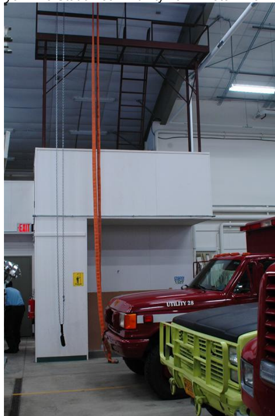
Kachemak McNeil Canyon Fire Station fire hose dryer rack. Photo: Brian Saylor, March 10, 2008. Alaska State Troopers and the forest service personnel often use the facility. Pat Johnson said that “people really appreciate the building. As more people see it as they drive-by, day will use it even more. It is like a bear is coming out of hibernation.” Facility Planning
