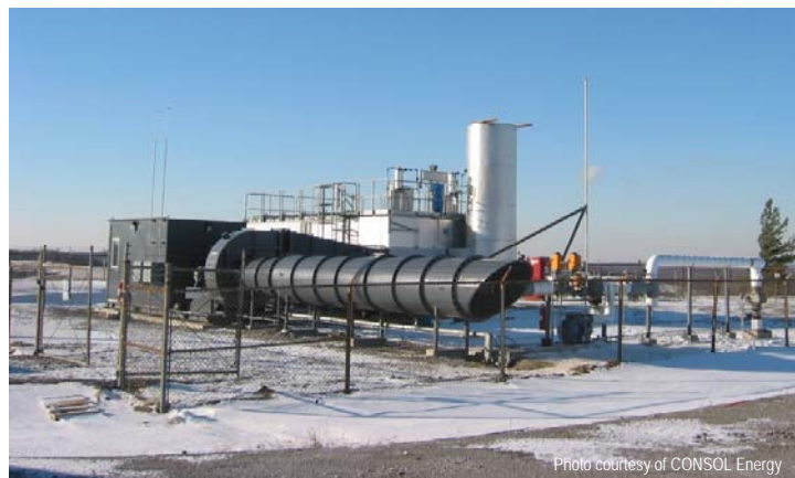
Figure 1. MEGTEC's VOCSIDIZER installed at CONSOL Energy's Windsor Mine Portal in West Virginia.
