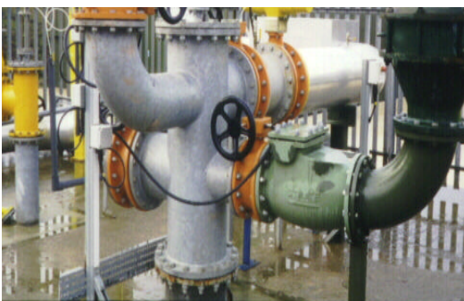
Gathering facilities at Alkane Energy's Steetly abandoned mine methane power project in Nottinghamshire, England. (Photo courtesy Raven Ridge Resources, Inc.)
