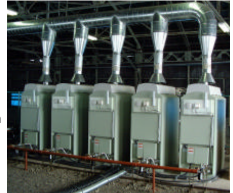
Five 30-kW microturbines use coal mine gas with a CH 4 concentration of 80% (photo courtesy Raven Ridge Resources, Inc.)
