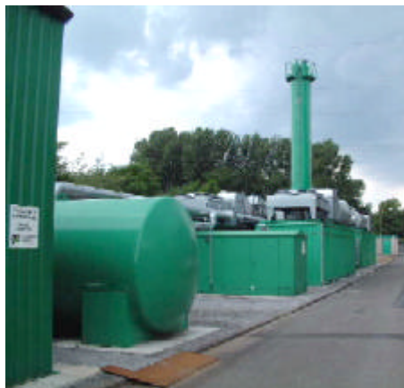
CMM-Fueled CHP Plant, Lunen, Germany Photo courtesy of G.A.S. Energietechnik
