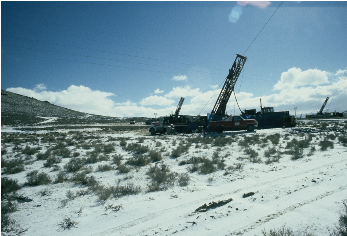
Development Drilling Defining the Extent of the Mineral Deposit at the Site That Became the Lone Tree Mine in Humboldt County, Nevada
