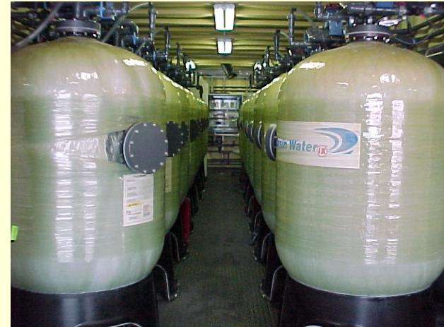
Central Water Treatment Plant
