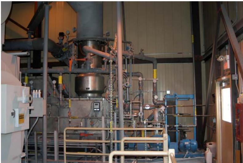
Figure 4 – RML Incinerator Scrubber System
