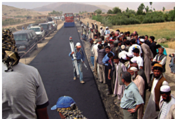
Road rehabilitation in Afghanistan makes goods and services more accessible to families and businesses, and allows local producers to sell to wider markets.
