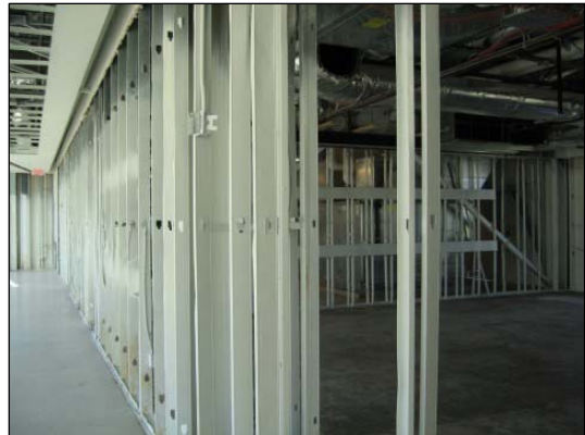
Construction to rebuild the estimated $500 million in damages at Dillard University is underway.
