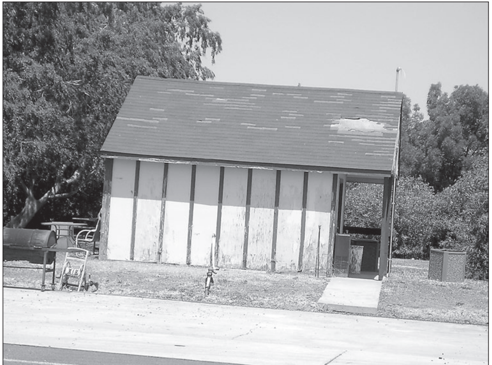
Figure 1: Dilapidated Maintenance Shed
