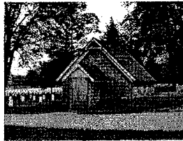
Abandoned, Deteriorating Old Caretaker's House
