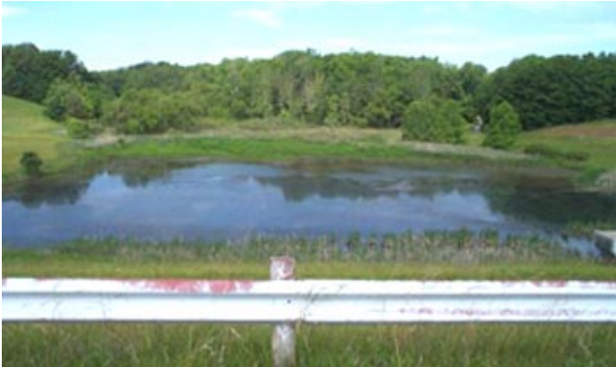
Upper Hocking Dam No. 8, looking upstream. The lake has filled with sediment reducing room for flood water storage.
