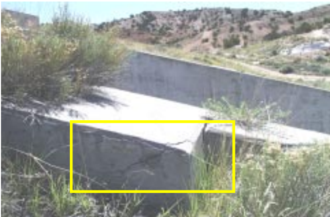
The concrete in the auxiliary spillway is experiencing severe cracking and is not expected to last much longer.
