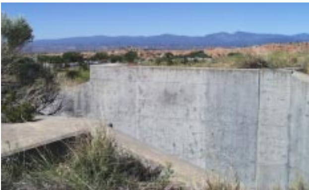
View from top of dam with the auxiliary spillway in foreground and homes downstream.
