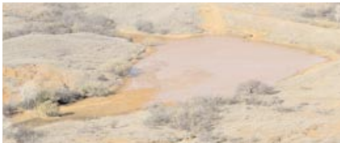
This lake has filled with sediment, has severe leakage in the principal spillway pipe, and the dam needs to be rehabilitated to protect homes downstream.
