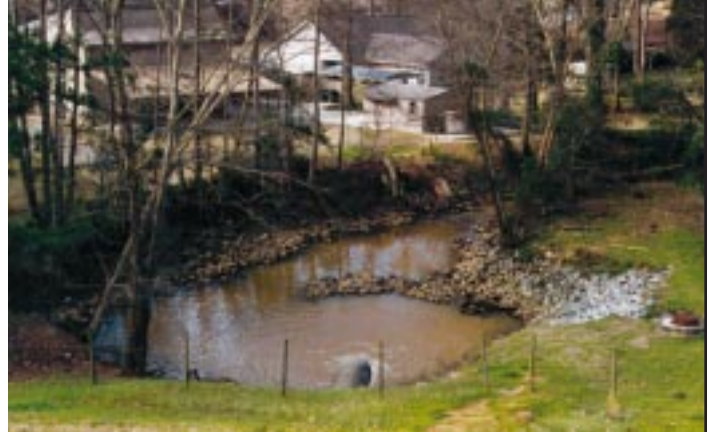
THE PROBLEMS. In Georgia, 121 dams need to be modified due to downstream development, which includes homes, buildings and a shopping mall. Other problems the dams face include sedimentation, spillway deterioration, eroding outlets, and malfunctioning and inoperable gates.
