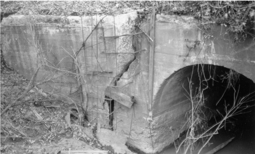
Cracked and displaced headwall at a bridge in Maryland on Amtrak's main line between Washington, D.C., and Philadelphia, Pennsylvania. Defects such as this can occur from repeated freeze and thaw cycles and can lead to deviations in track surface or alignment. The complete failure of an embankment structure can result in a total loss of service on a line.
