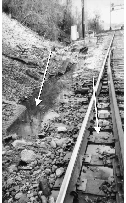
A section of Northeast Corridor main line track at an interlocking in Philadelphia, Pennsylvania, along Amtrak's Harrisburg line. The arrows indicate poor water drainage that, according to Amtrak, is illustrative of conditions existing at various locations on the Northeast Corridor. An inability to maintain adequate drainage can ultimately weaken track structure and lead to deviations in track surface or alignment that must be corrected or speeds reduced.
