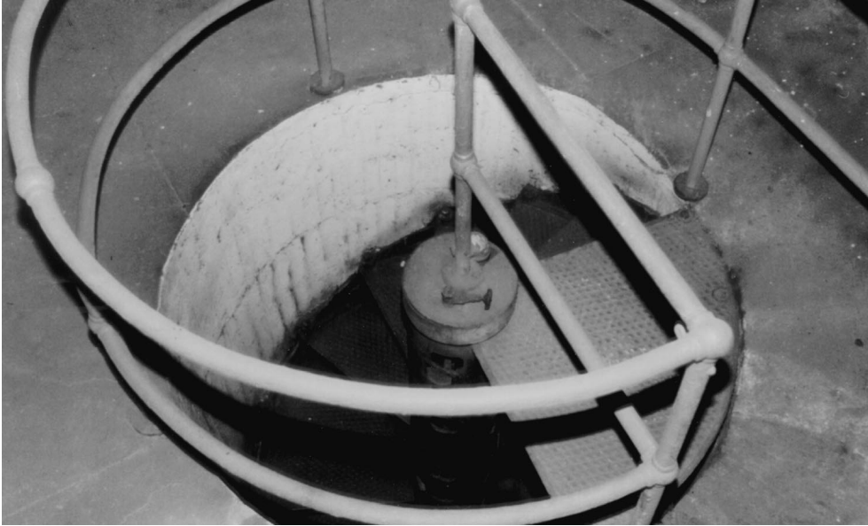
Figure 9: Illustrations of Current Infrastructure Conditions on Amtrak's Northeast Corridor
