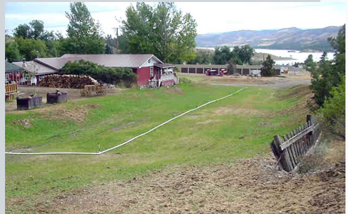
Now, a dike in front of the home helps keep flood waters and debris away from the home. Homeowners are using water from the stream, which has been redirected, to help grass establish in the channel.
