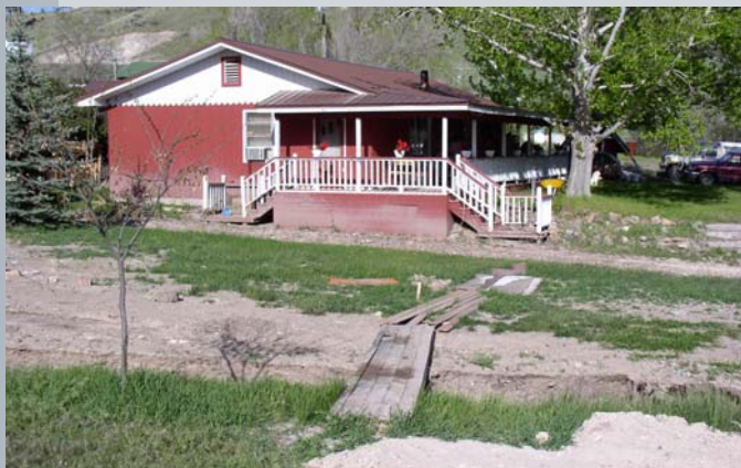
This home sustained damages from flood water. Water marks on this home (the gray area on the walls) show how high water rose during some of the flood events.
