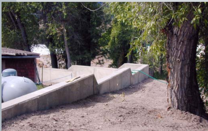
Concrete barriers were used to protect property where there was limited room to build a dike and/or channel.
