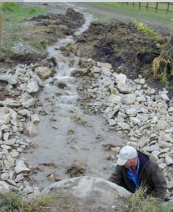
Left: Highway 284 sustained damage when water and debris were forced to flow over the road because the small culvert was too small to handle the flows.
