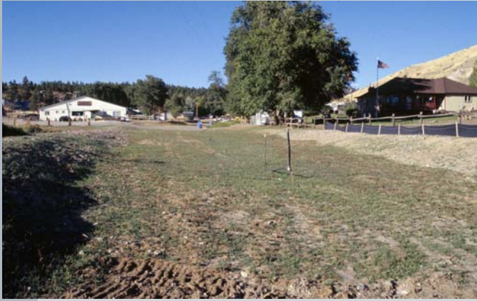
Above: The dikes, grass, and covered geo-grid material filled with rock armoring a little further upstream of Highway 284.
