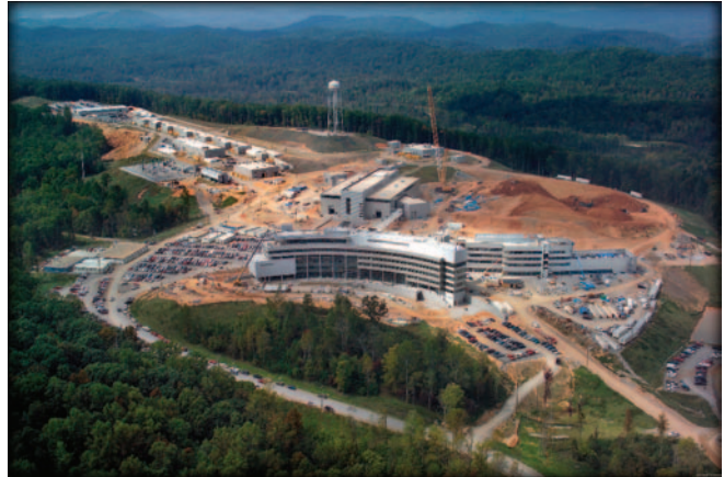
The $1.4 billion Spallation Neutron Source at Oak Ridge National Laboratory in Tennessee will provide the most intense pulsed neutron beams in the world for scientific research and industrial development.
