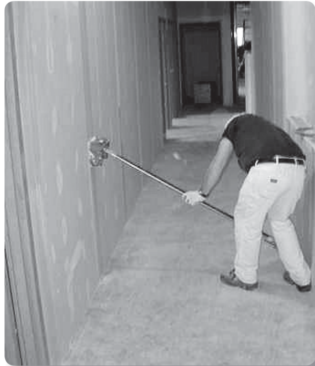
Problem: Hand drywall finishing with mudbox
