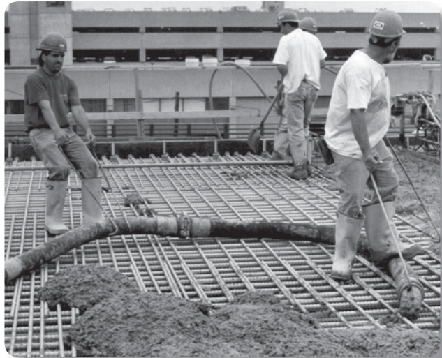
Problem: Pulling concrete hose without skid plate
