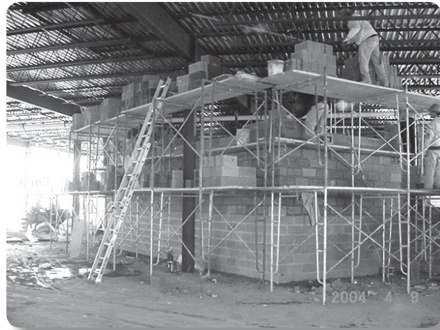
Problem: Conventional unguarded frame scaffolding
