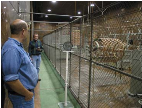
Photo 5: E-Field measurement located in the Combiner Room Entry (Copper Room) near the T-15 switch
