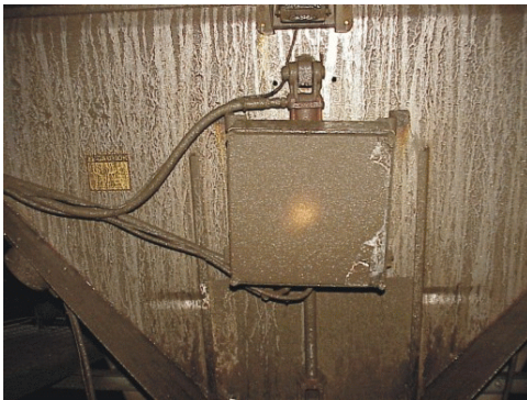
Figure 12.—Mud build-up on radar enclosure.
