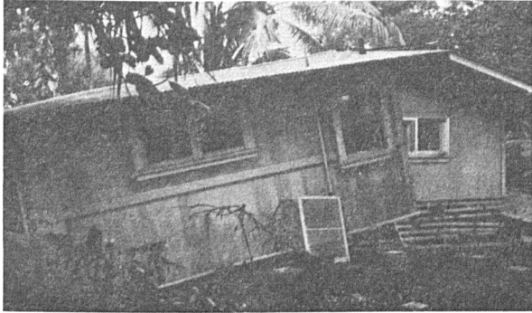
FIGURE 22.—Damage to small home in Reeds Bay area near Hilo, Hawaii, from the tsunami of November 4, 1952. Note foundation blocks from which building was lifted. (Photo Credit: National Oceanic and Atmospheric Administration)
