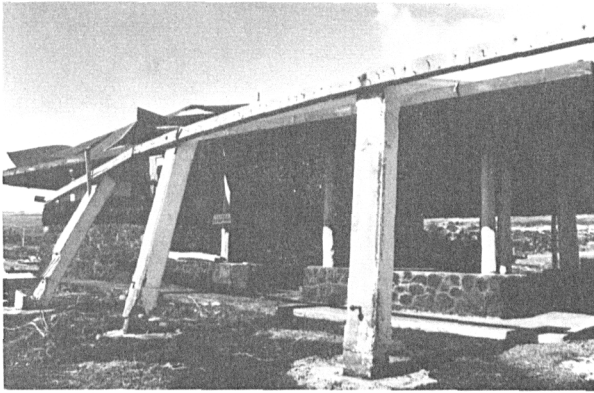
FIGURE 30.—Structural damage to restaurant and gift shop at Punaluu, Hawaii, as a result of the tsunami of November 29, 1975. (Photo Credit: International Tsunami Information Center)
