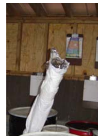
Photo 1: Drainage pipe with radioactive scale.
