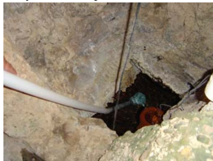
Photo 9: Natural spring in the basement of the Hale Bathhouse. The white pole was used to obtain the water samples.
