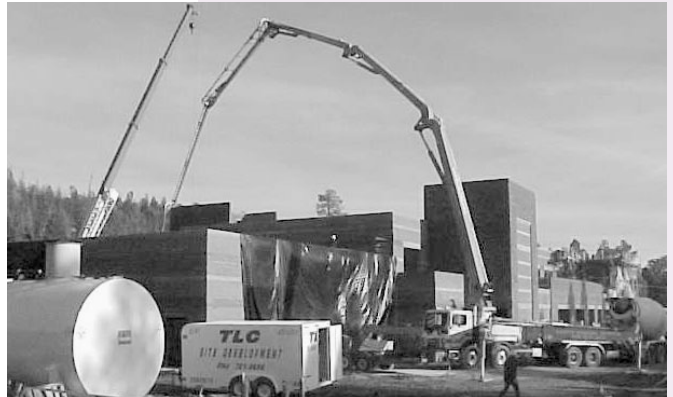
A concrete pump truck pours the roof of the new EOC, while the crane in the background places electrical equipment. The underground utilities subcontractor, the TLC company, installed the water line in the location where it will connect with the emergency fire protection water tower tank.
