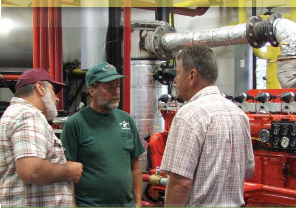
Vermont dairy producers Brian Rowell (center) and Bill Rowell (right) check on the on-farm generator that produces electricity from a manure-to-methane gas digester on their Green Mountain Dairy Farm. Photo courtesy University of Vermont Cooperative Extension
