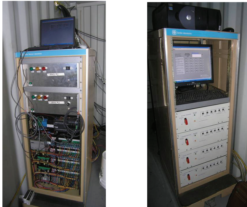
Figure 3.11: Photograph of the IRMS (left) and SCDU racks.
