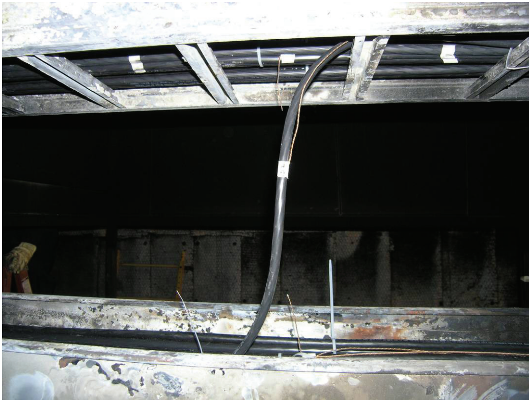
Figure 6.24: Photograph of the air drop cable in IT-2.
