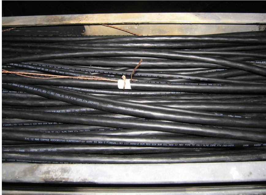
Figure 6.18: Photograph of the random fill cable tray at Location A in IT-1.
