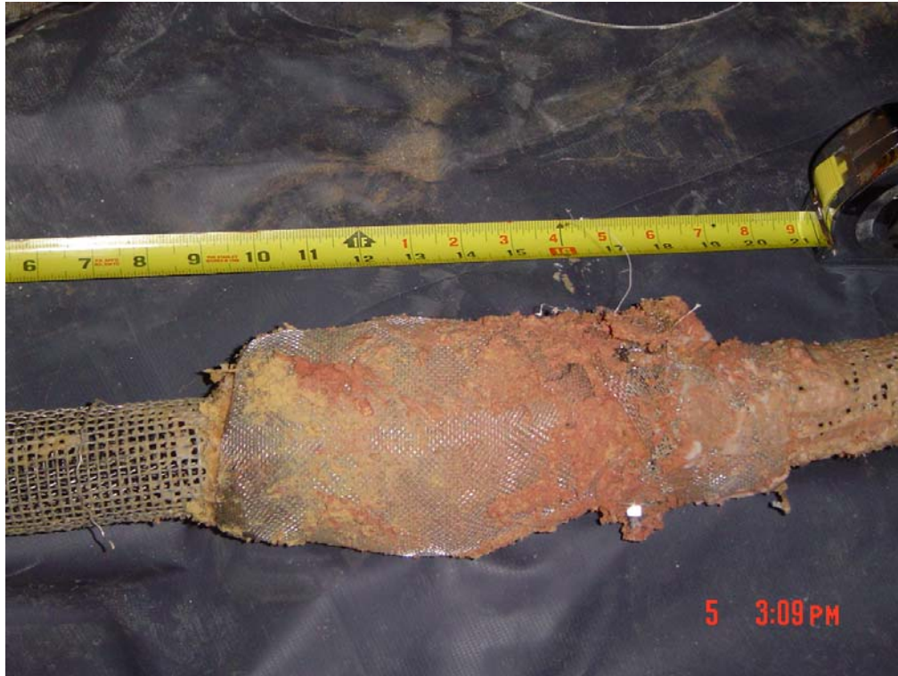
Figure 3-60. Drain screen collar removed from the tank.
