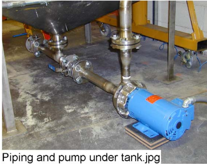
Figure 12. Circulation pump for the ICET system.
