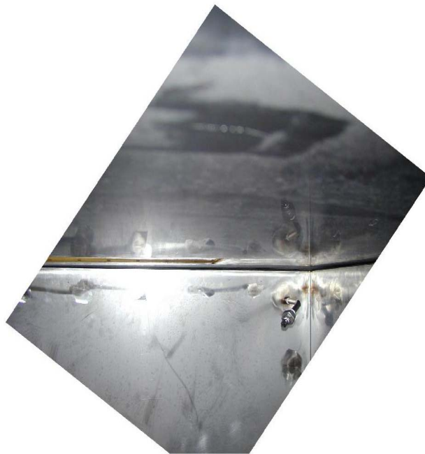
Spray nozzle inside tank.jpg
