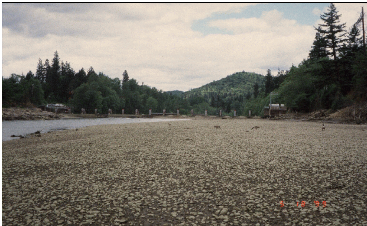
Photograph 9.— Savage Rapids Dam, Rogue River Basin Project, Oregon. View downstream toward Savage Rapids Dam showing the exposed surface of the north bar during stoplog installation on the spillway crest. This photograph shows the coarse-grained character of the sediments composing the north bar, which consists of variably mixed sand and gravel with cobbles. The volume of cobbles was field estimated at about 20 percent by volume at the upstream end of the bar, grading to about 5 percent at its downstream terminus at the spillway. This photograph shows the surface conditions near the approximate midpoint of the north bar. (Reclamation photograph by Richard Link; May 18, 1999.)
