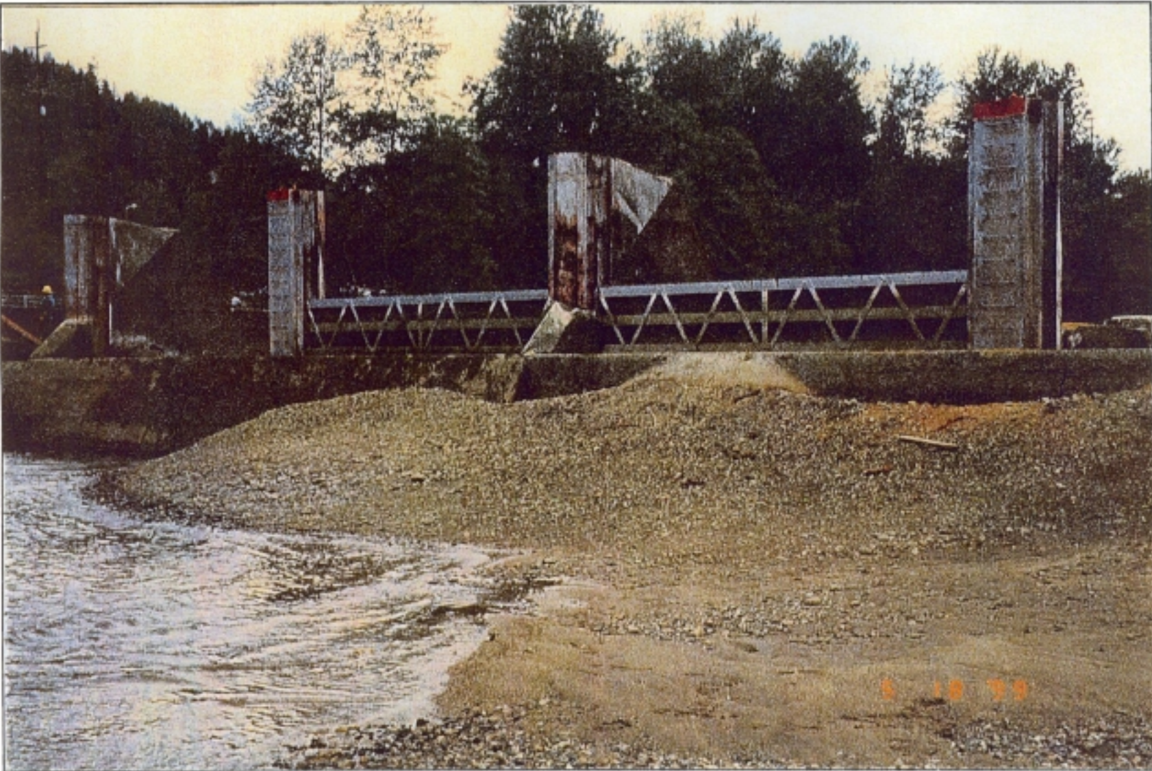
Figure 13. - Upstream face of Savage Rapids Dam - During a reservoir drawdown in May 1999, gravel-sized sediment was observed on the crest of the dam, indicating that sediment is transported past the dam during spillway releases.
