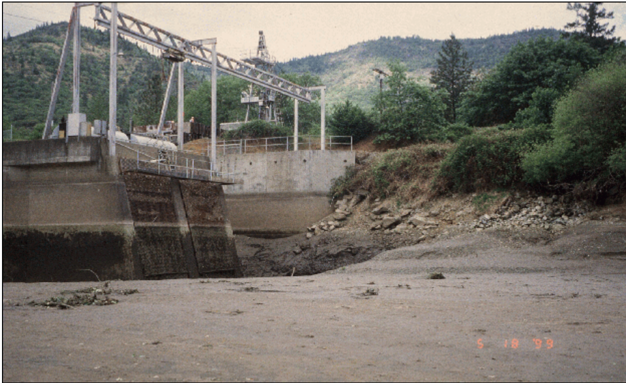
Photograph 7.—Savage Rapids Dam, Rogue River Basin Project, Oregon. View toward the north abutment of the dam and the pumping plant showing the conical depression formed in the surface of the north bar as a result of operation of the plant intakes. The reservoir is drawn down below the normal operational level to permit stoplog installation. Much of the surface of the north bar consists of a thin veneer of fine sand and silt which is similar to that observed upstream on the left shoreline at the south bar. (Reclamation photograph by Richard Link; May 18, 1999.)
