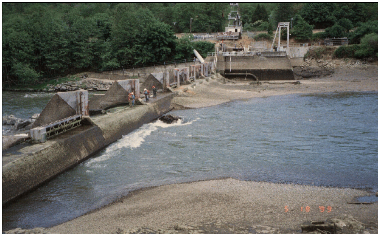
Photograph 6.— Savage Rapids Dam, Rogue River Basin Project, Oregon. View across Savage Rapids Dam toward the north bank showing the reservoir drawn down for installation of stoplogs across the spillway of the dam. Sediment has infilled the reservoir to the point that the north bar is lapping onto the concrete spillway, as can be seen in the distance, adjacent to the pumping plant. The bedrock outcrop forming the right abutment of the low-level radial gate outlet is exposed near the center of the photograph. (Reclamation photograph by Richard Link; May 18, 1999.)
