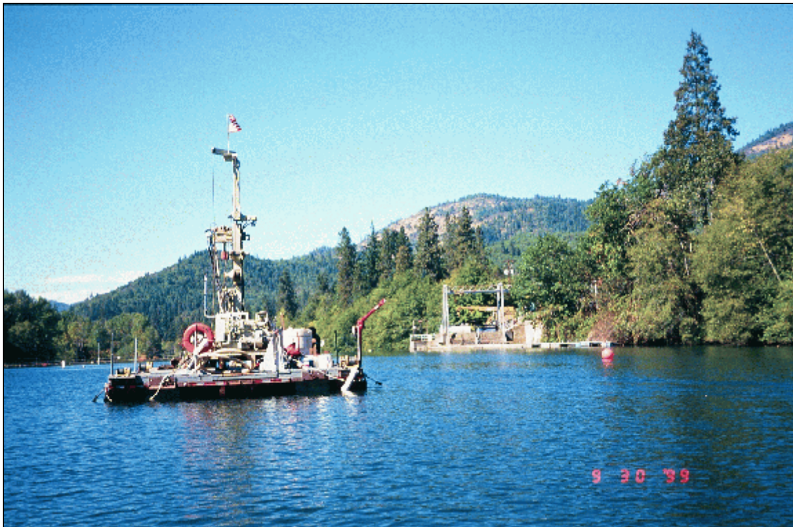
Photograph 1.—Savage Rapids Dam, Rogue River Basin Project, Oregon. View downstream showing Reclamation's custom built, floating drilling platform in operation on drill hole AP-99-10. Drilling equipment consists of a skid-mounted Ingersoll-Rand T200 rotary drill, which was used to advance 10-inch outside diameter, hollow-stem flight augers to a bottom depth of 27.8 feet below the lake surface in this hole. The spillway and pumping plant portions of Savage Rapids Dam are present in the background of this photograph. (Reclamation photograph by Richard Link; September 30, 1999.)
