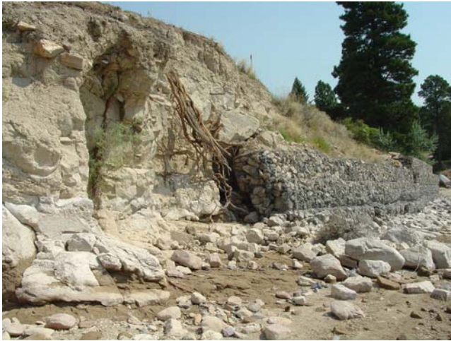
Figure 8. An example of a gabion wall on Canyon Ferry Reservoir with flanking erosion due to deflected wave energy.
