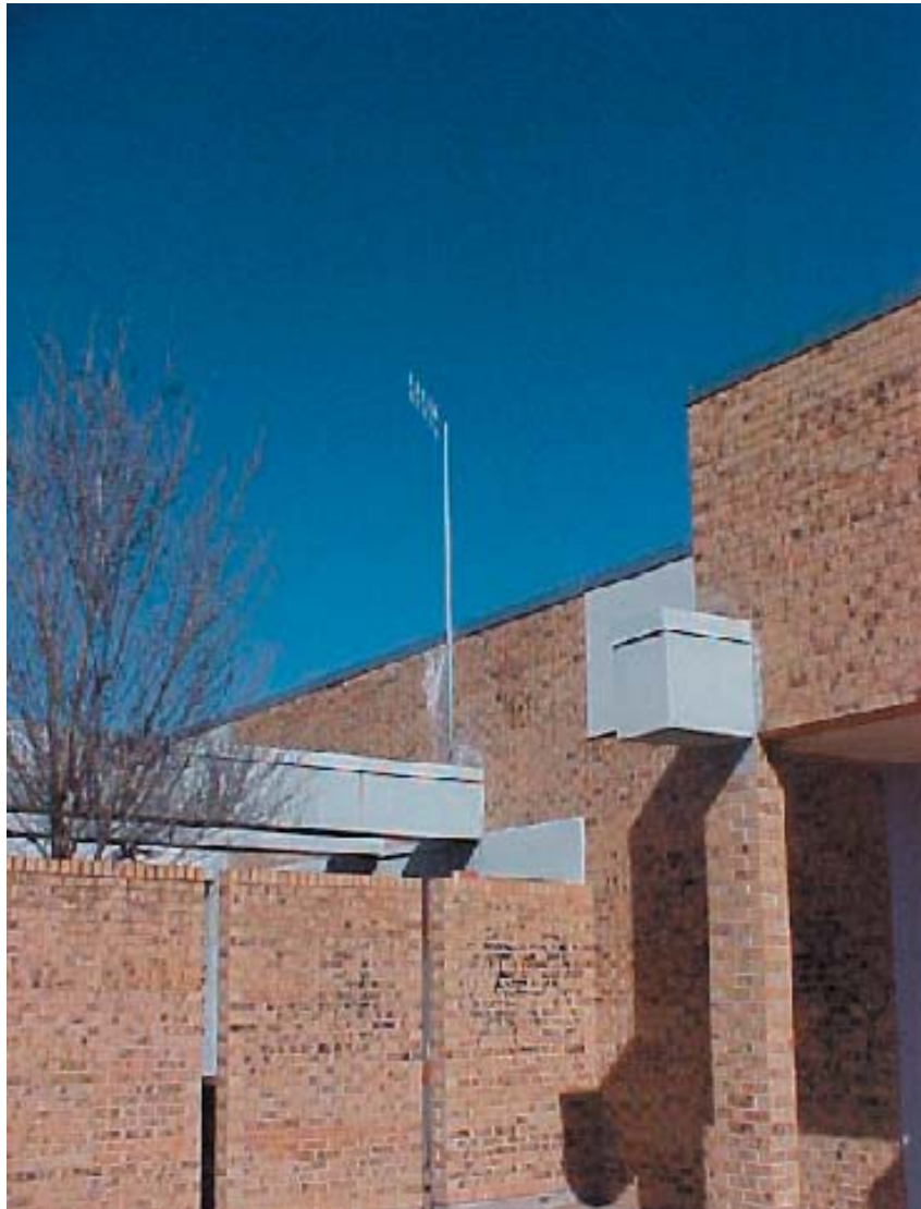
The signal from the measurement site is received approximately 15 miles away via a not-line-of-site path using a small antenna atop the Lower South Platte Conservancy District Office.
