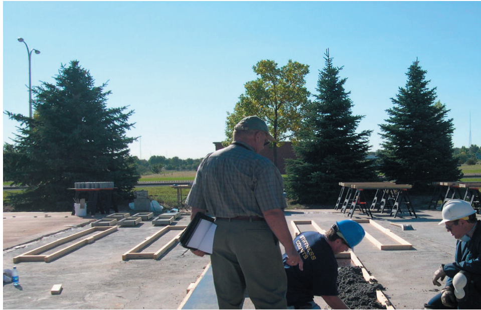
Placing repair materials for phase 2 testing. Placing materials in long, narrow shapes like this is a key element of this phase.
