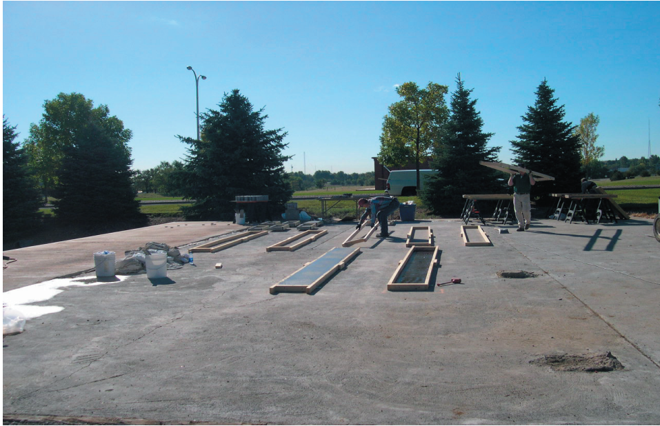
Final preparations of the site for the phase 2 test program on the Denver Federal Center.
