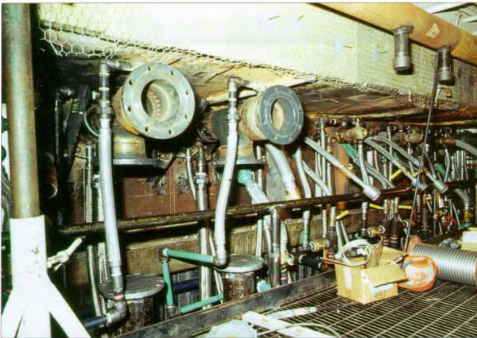
Natural gas injectors being installed at Lakeside. Flanged piping is for connecting recirculated flue gas lines.
