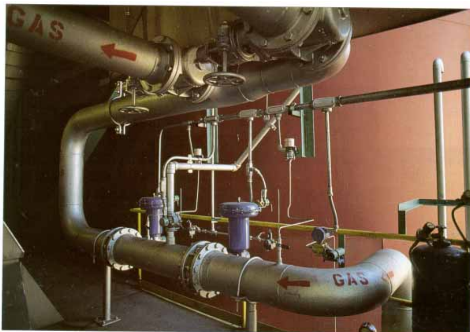
Main process gas supply.
