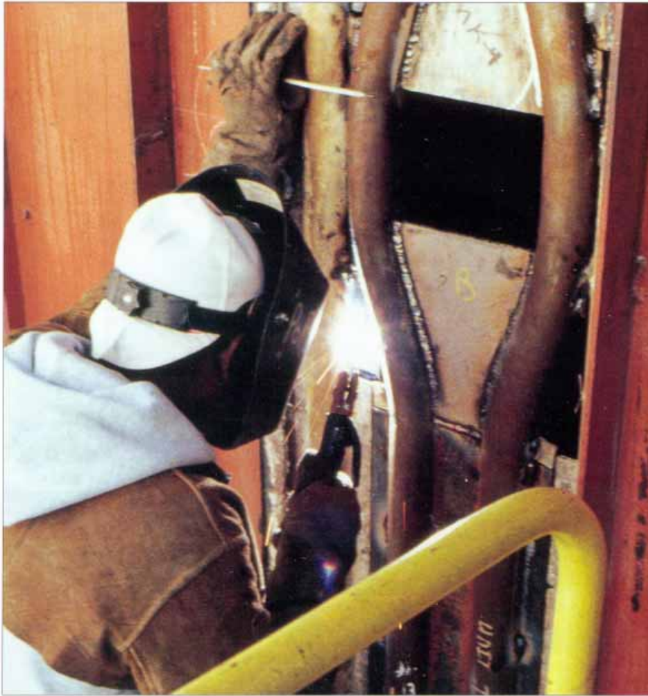
Shaped boiler tubes, part of the over-fire air and gas reburn system, were welded into the boiler wall at Cherokee Station.
