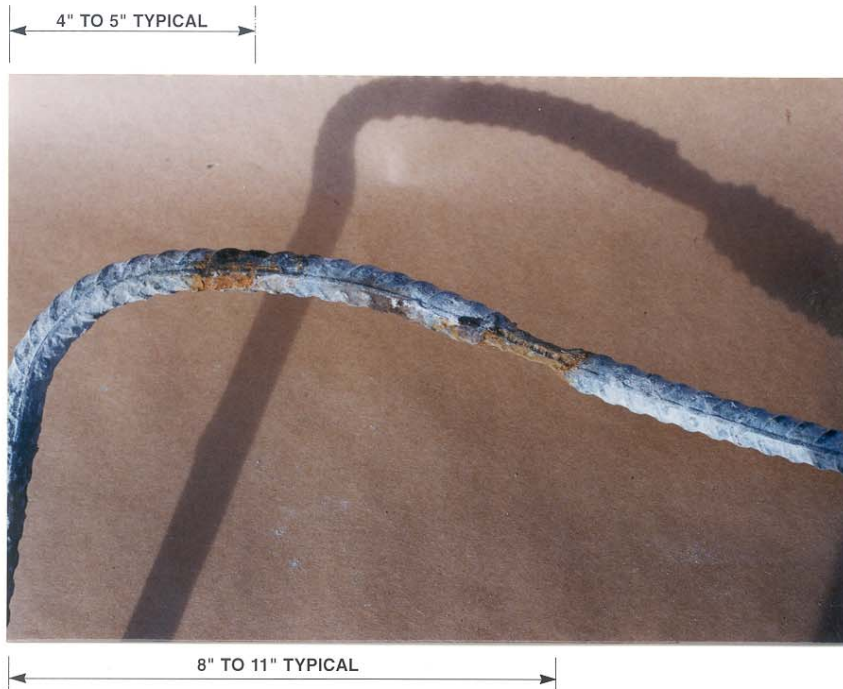
Photo 3.3 Dowel "A" showing corrosion at two locations.
