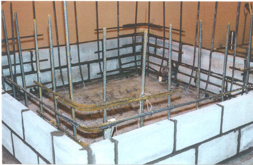
Photo 3.10 Concrete foundation slab with dowels and first two courses of insulating block.
