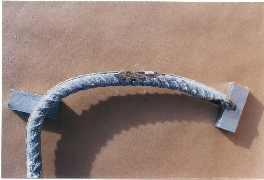
Photo 3.7 Dowel "D" showing corrosion at two locations. Vertical portion of dowel broke off during demolition.
