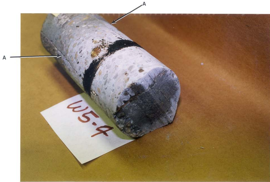
Photo 2.13 Crack "A" appears to be a parting line between concrete pours due to the presence of mastic sealant placed between pours.
