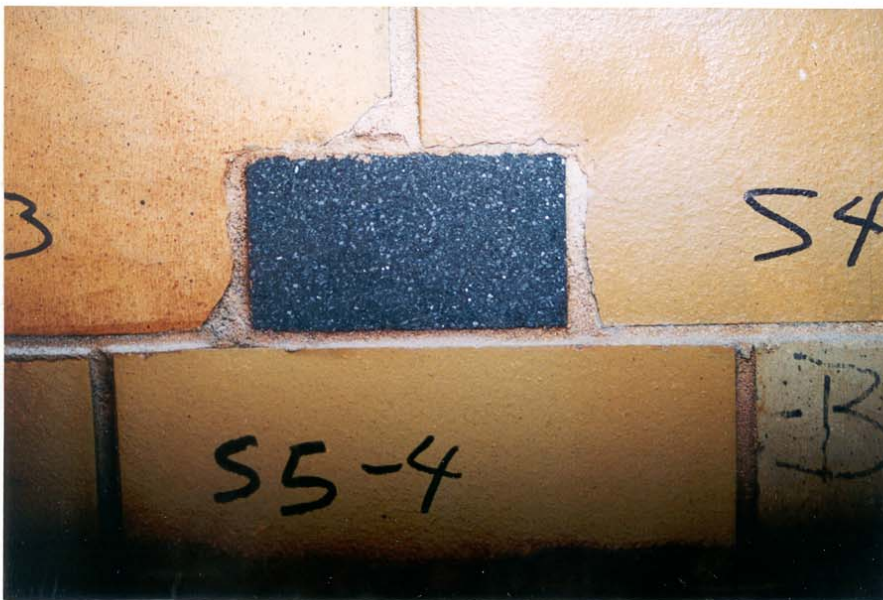
Photo 1.8 "Refrax" plug on south wall shows grout to be in good condition. This plug was located in a spray impact area above the normal slurry level.
