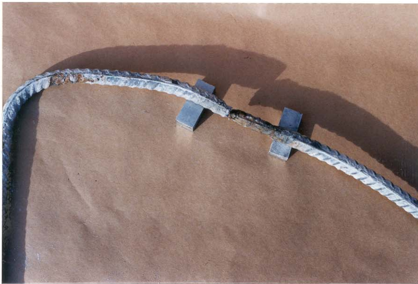
Photo 3.8 Dowel "E" showing corrosion at two locations. Vertical portion of dowel broke off during demolition.
