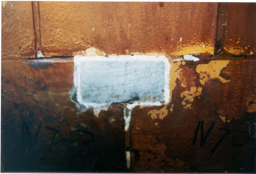
Photo 1.7 "Refrax" plug on north wall shows grout to be in good condition after scale had been scraped off. This plug was located below the normal slurry level.
