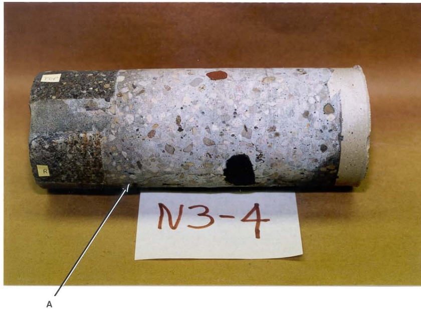
Photo 2.4 Crack "A" appears to be a parting line between concrete pours due to the presence of the mastic sealant normally applied to the previous pour.
