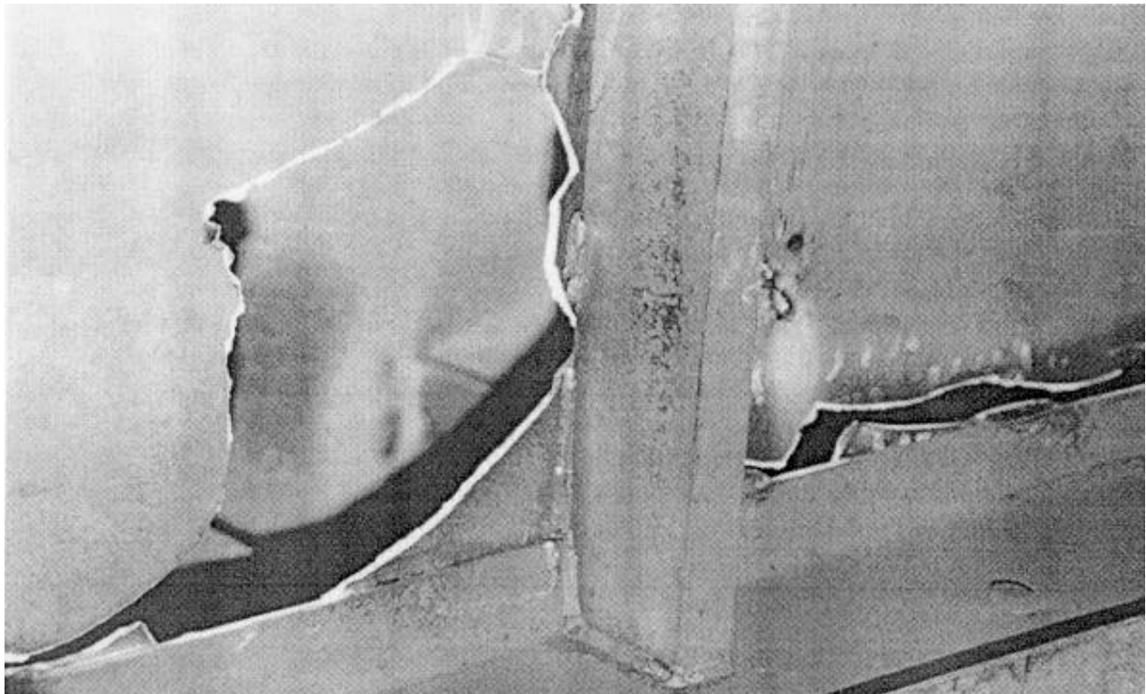
FIGURE 4.11-13 VIBRATION DAMAGED DUCT BETWEEN THE 2A HEAT PIPE OUTLET AND THE PRECIPITATOR INLET
