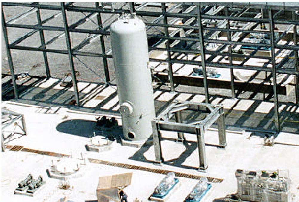
Figure 7 - "Tabletop" for Reactor Mounting
