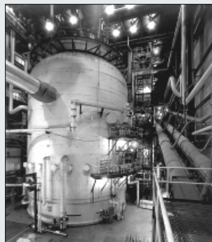
Pressure vessel is shown fully installed with insulation on exposed surface
