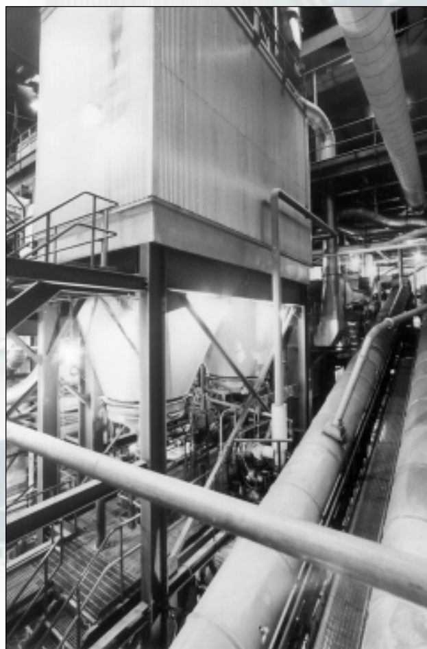
Sorbent silos with coal and sorbent conveyors to the right.
