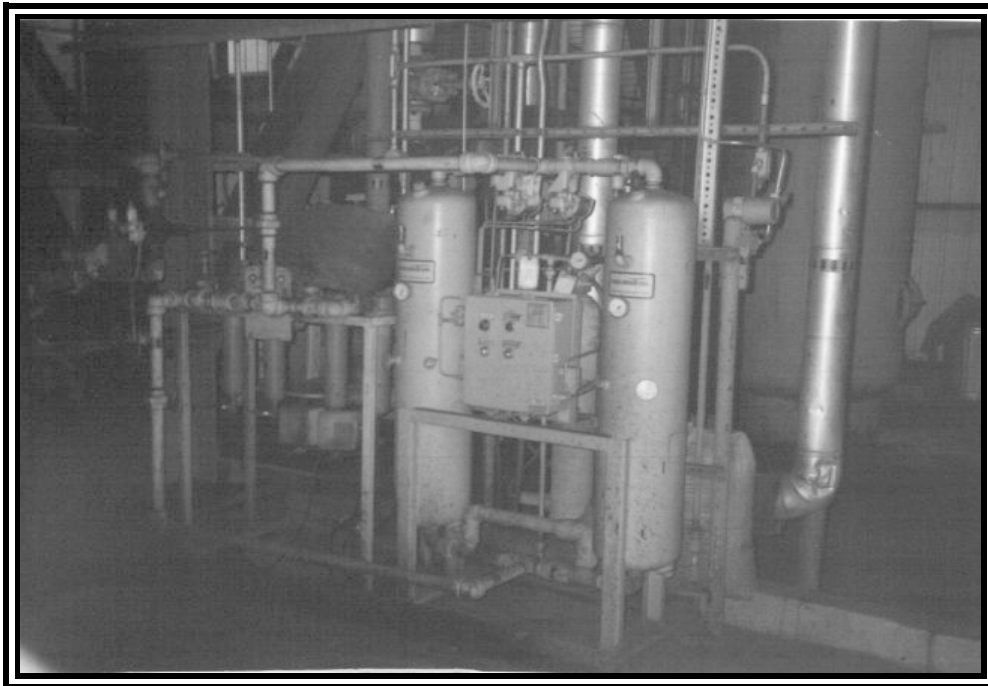
Figure 5.2: Instrument Air Dryer.
