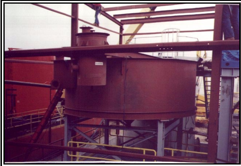
Figure 5.8a: Process Water Clarifier.
