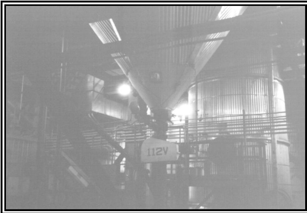
4.3b: Pyrolyzer Cyclone Fines Discharge.
