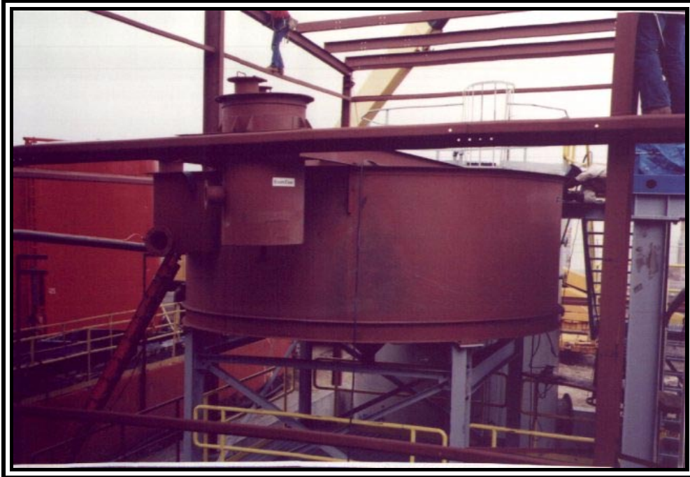
Figure 5.8a: Process Water Clarifier.
