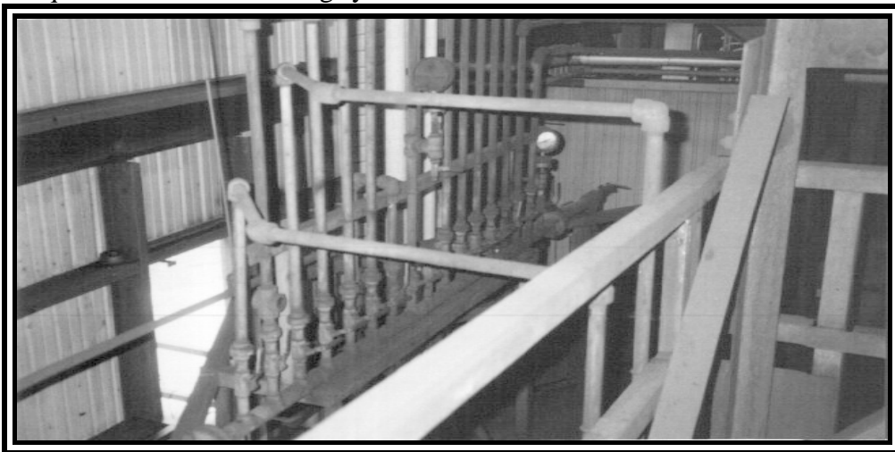
Figure 4.4a: Pyrolyzer Quench Table Water Supply Header.
