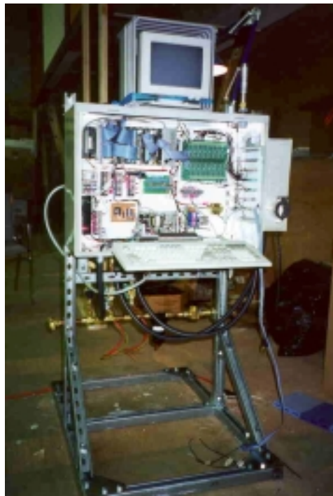
Figure 2 CAM Carbon-in-Ash Monitor (Interior View)
