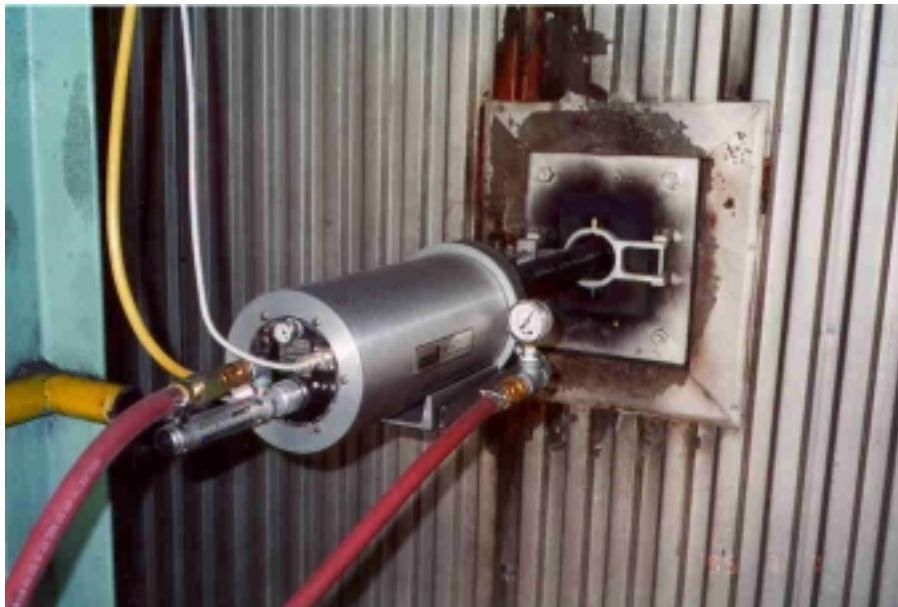
Figure 2 FOCUS Camera Attached to Furnace Inspection Door
