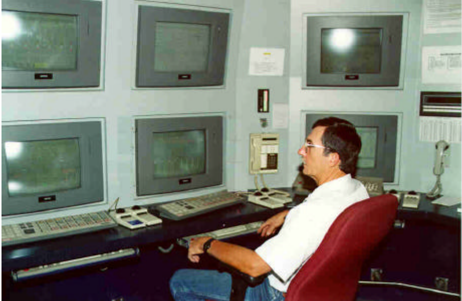
Figure 2-5 Photo of Unit 4 Benchboard
