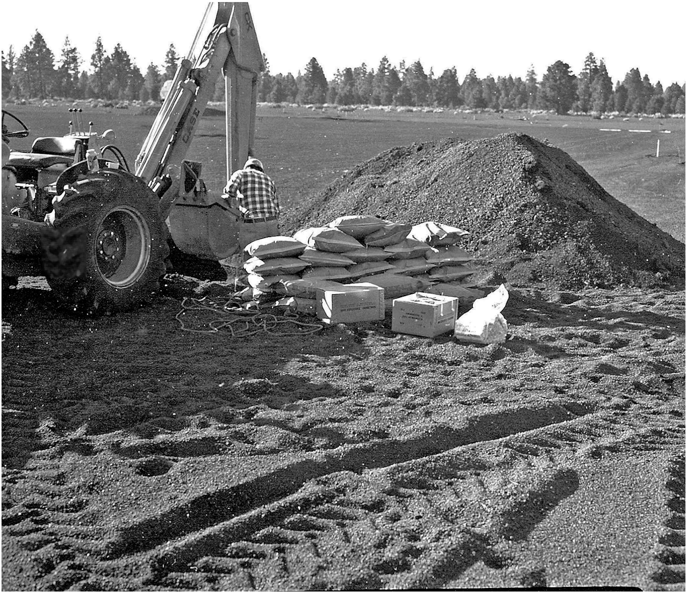
Figure 48-(b) loading of holes with dynamite (312.5 pounds) and ammonium nitrate (13,492 pounds) (trade name Nitro-Carbo-Nitrate; mixture of common agricultural fertilizer and fuel oil) (l-r) unknown, George Ulrich and Red Bailey; USGS photo P447, F106757
