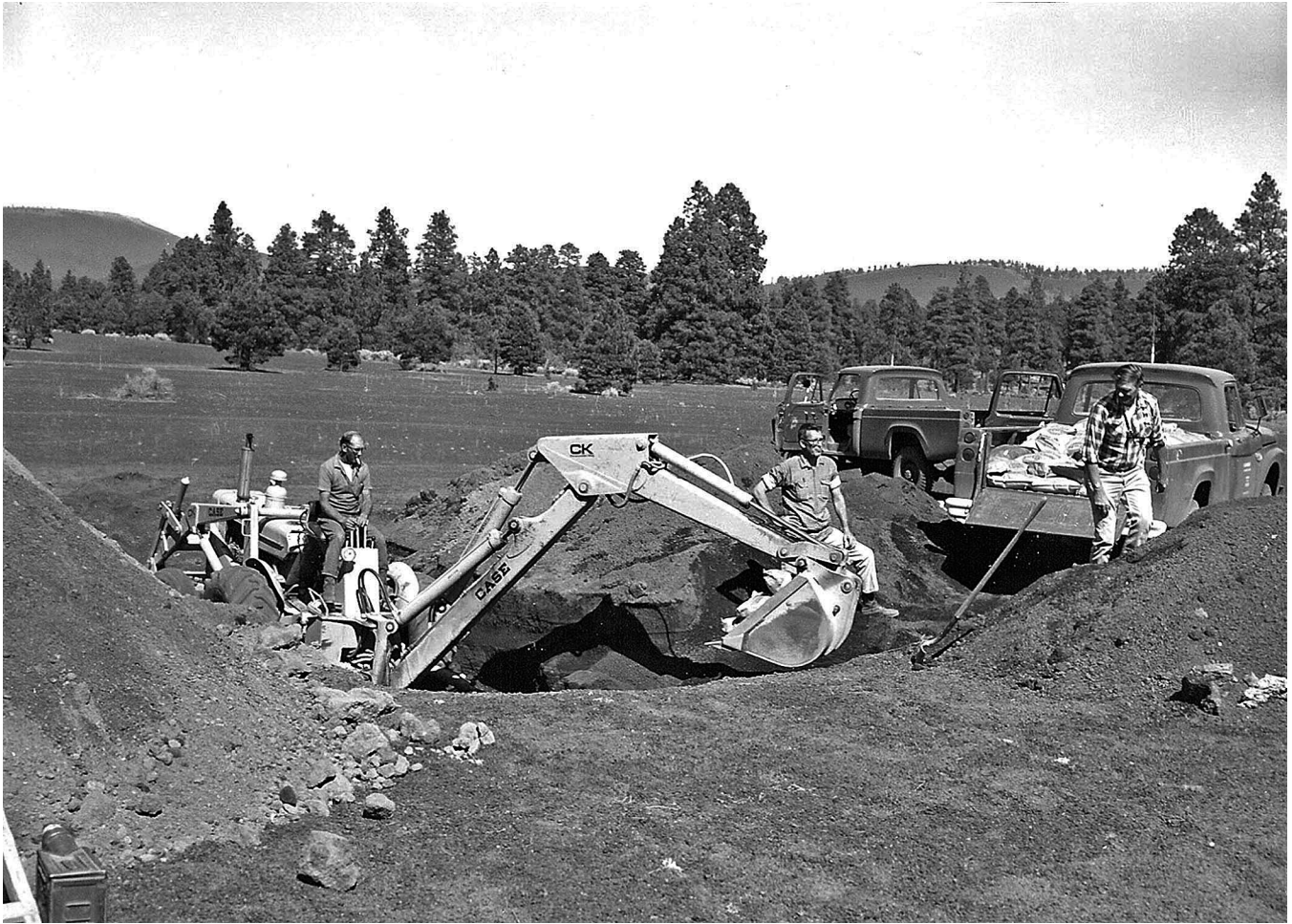
Figure 48-Construction on 27-28 July 1967 of Cinder Lake Crater Field # 1 just northeast of Flagstaff, Arizona (a) backhoe digging of 47 holes to precise depths, and in which to bury precisely-measured explosives at each surveyed crater site; red bailey back to camera P447, F106754
