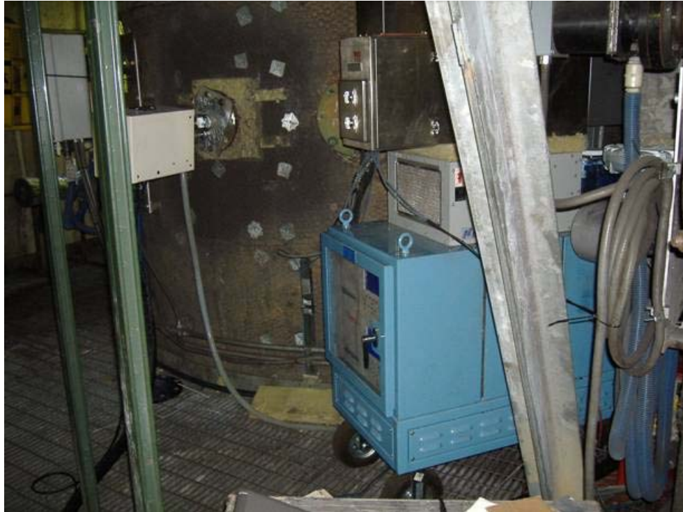
Figure 1. Portable IRM Installed at 200' Level in the Stack
