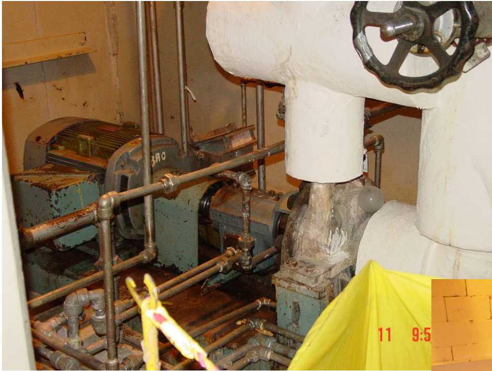
Reactor Water Cleanup Pump 1A Elevation 593 December 2002
