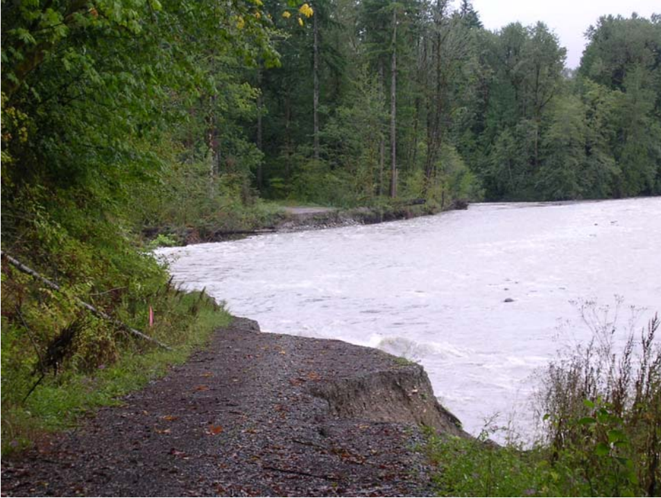
Photo 1. North Sauk River Road washout from downstream end looking upstream.
